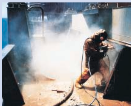
Spot repair and surface preparation on deck with the 3000-bar Modular Gun System .
