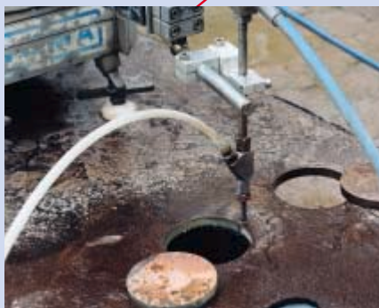
On-site cutting of openings in walls and ceilings with the 3000-bar circular abrasive cutter Eco Top Cutter 3000 .
