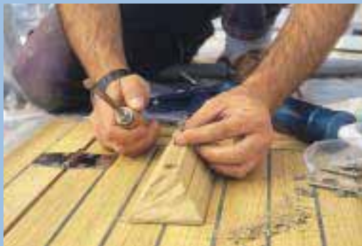
Teak deck repairs and replacement, incorporating both traditional techniques and the latest in pre-fabricated deck sections, dramatically cutting down installation time.
