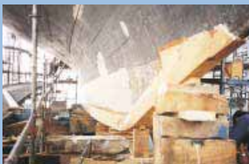
Wooden hull repair and maintenance, here involving replacement of part of the keel section and stern post.
