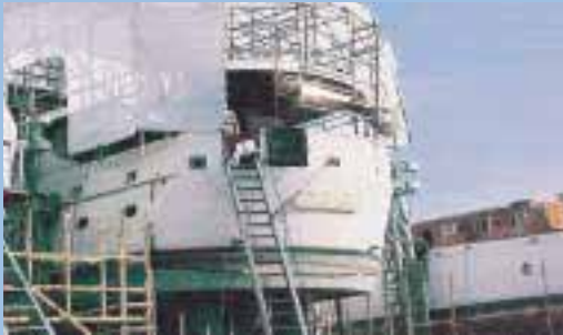
Steel hull extension for M/y Shark. The old stern was completely removed and replaced with new extension for extended lazarette and machinery space.
